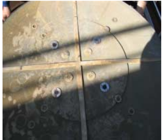
Figure 6: Typical HFO ash deposited on the catalyst
