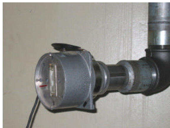
(d): The high volume PM sampler fitted to the pipe terminal
